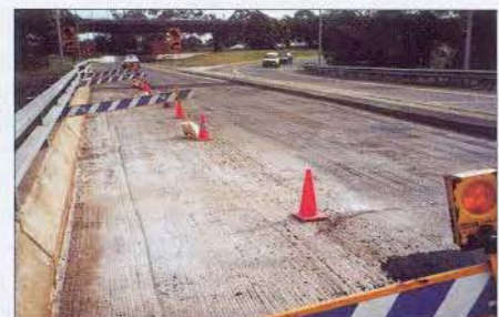
FIGURE 14 - SCABBLED BRIDGE DECK
