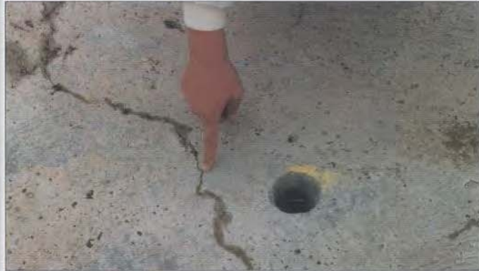
FIGURE 16 - CRACKING IN CONCRETE
