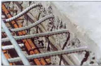
FIGURE 11 - EXPOSED CONSTRUCTION JOINT
