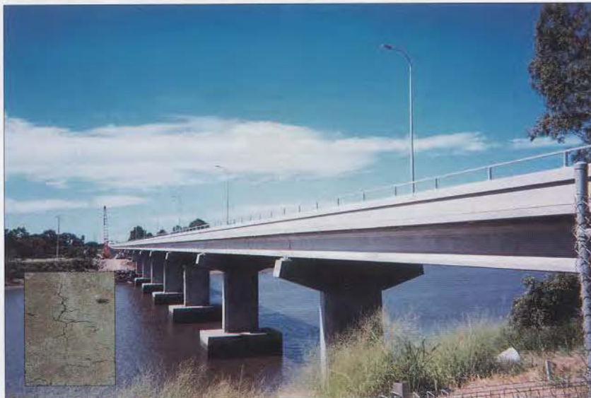
FIGURE 1 - NEW BURNETT RIVER BRIDGE WITH CRACK INSERT
