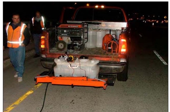
Pictured above: RADCON Formula #7 application - electrical pump/tank with a hose spray wand or a boom with a number of sprayers.
