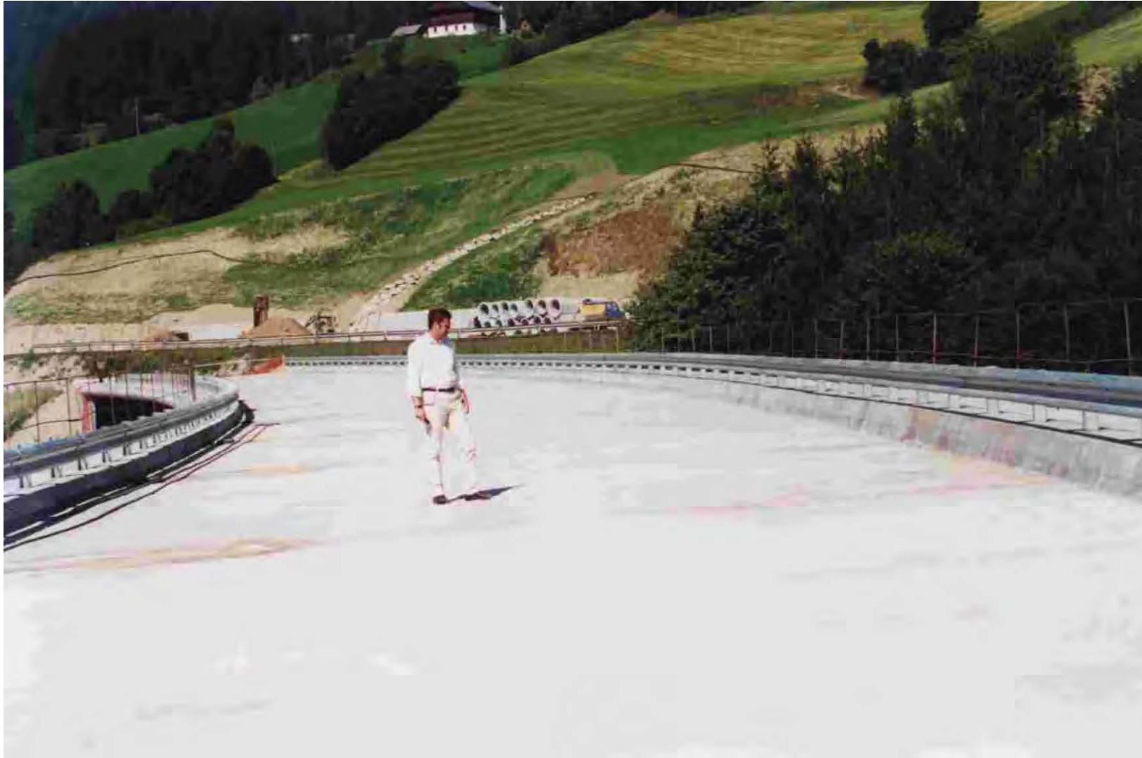
Bridge of MONGUELFO highway, (BOLZANO) - 2.500 Sqm Waterproofing with RADCON #7 of the bridge deck.
