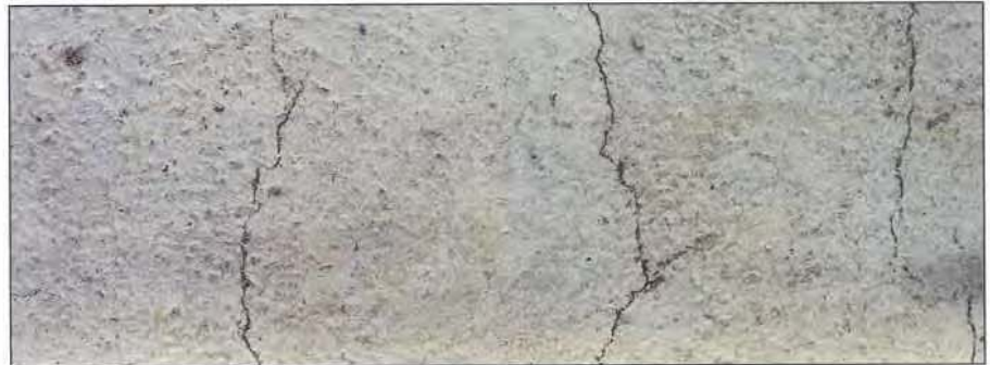
SEVERE CRACKING IN SLAG BEND - EVIDENT
